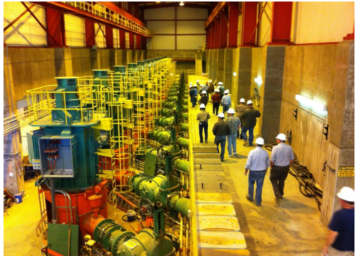
Visitors tour the inside of the Pacheco Pumping Plant, located near the San Luis Reservoir about 24 miles east of Hollister over the Pacheco Pass. The 12 large pumps in the left of the photo pump water west through the Pacheco Tunnel and Pacheco Conduit, where it is then diverted into the Hollister Conduit and the Santa Clara Conduit.
